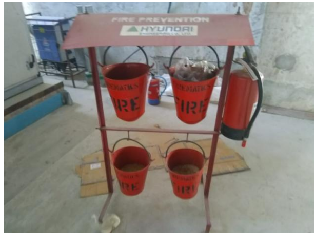
Figure 2.4. Fire Fighting Facility
