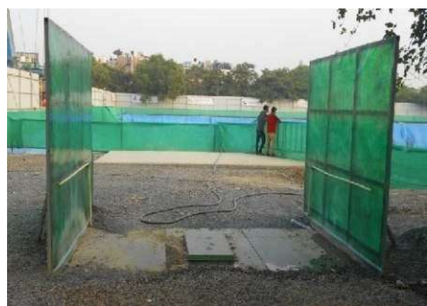
Figure 2.4. Wheel Wash Facility
