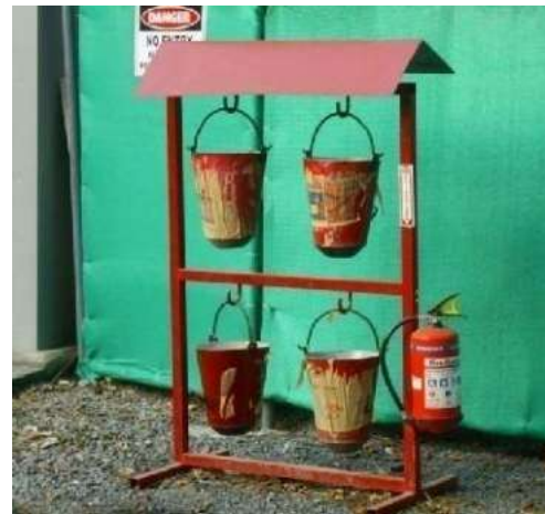
Figure 2.2. Fire Fighting Facility
